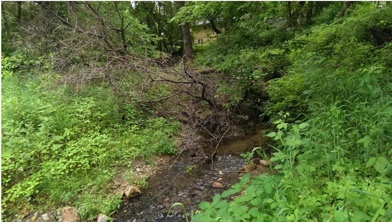
Photo 2: Stream section facing upstream directly behind garage (sudden drop-off on the right caused by recent erosion, new plant growth on the left, and a previously fallen tree caused by stream bank instability)
