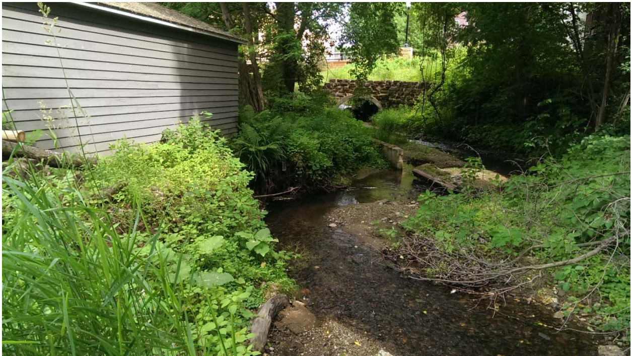
Photo 8: Downstream section of stream with significant erosion encroaching on the garage and damaged retaining wall
