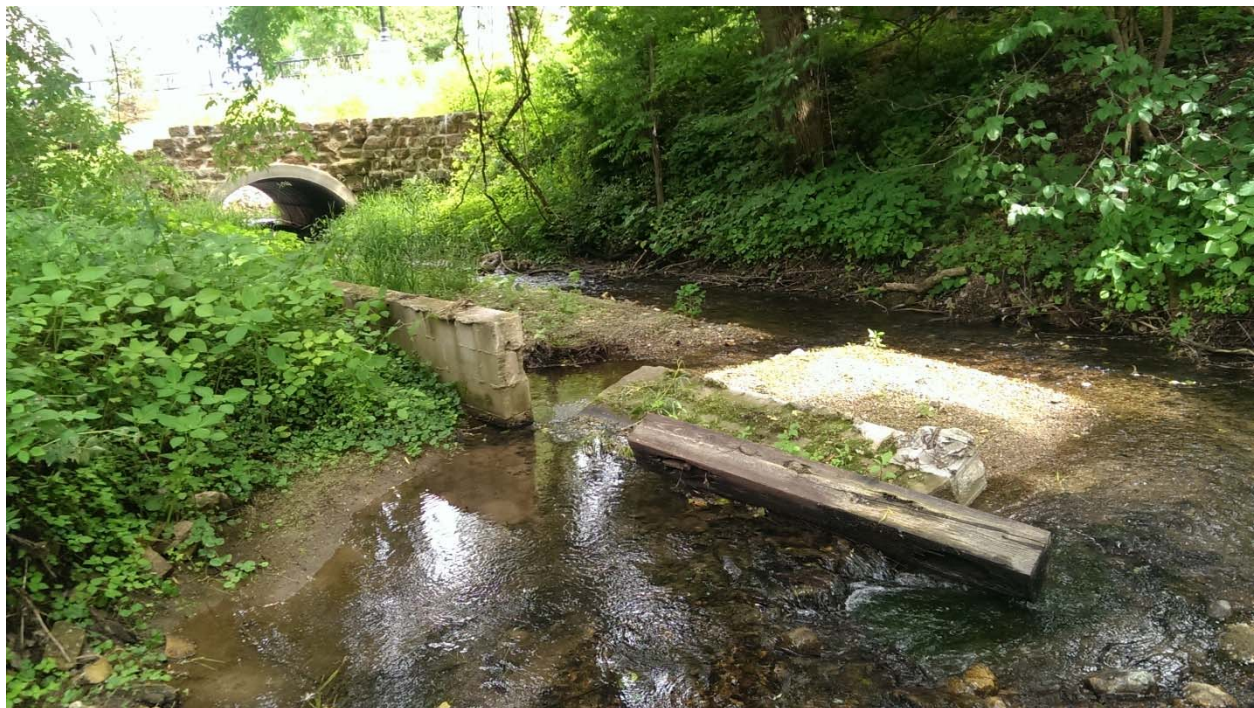
Photo 10: Close-up of damaged retaining wall most likely caused by stream path change
