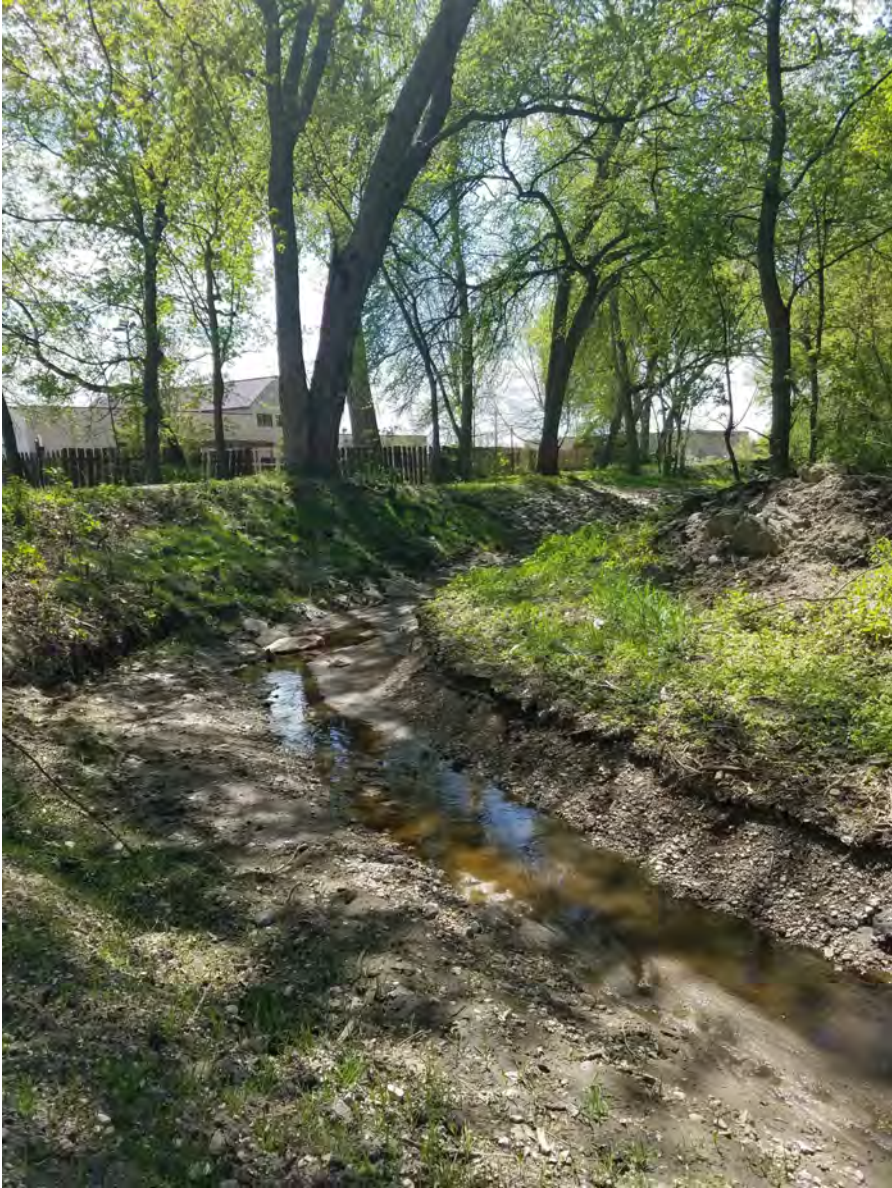
May 6, 2021—Looking downstream at right bank spoils pile and poor vegetation establishment before final grading.
