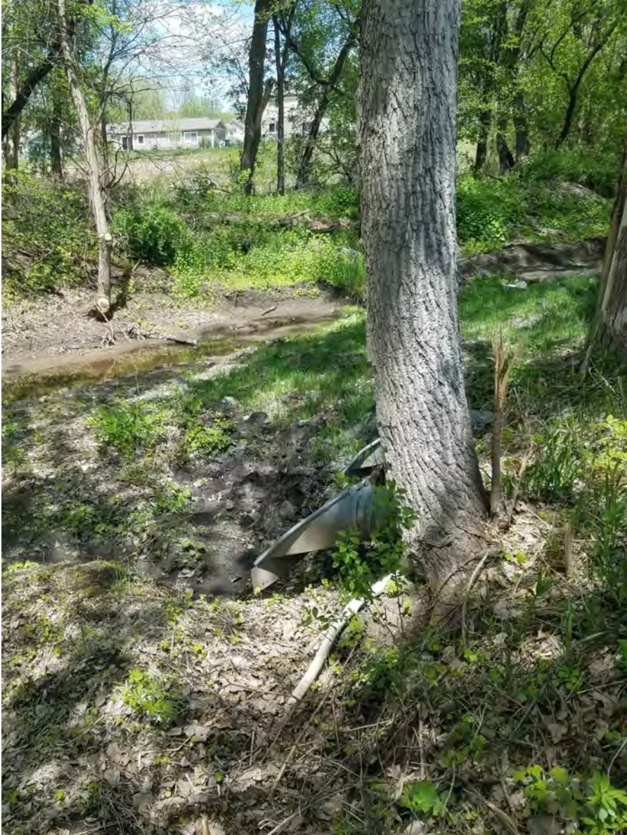
May 6, 2021—Hanging pipe outfalls outside the project limits.
