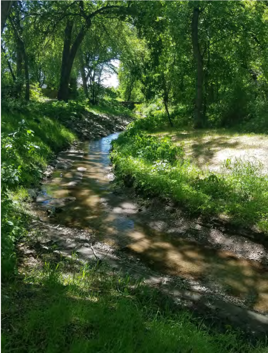
May 28, 2021—Spoils pile removed and erosion control blanket and seeding provided on right bank
