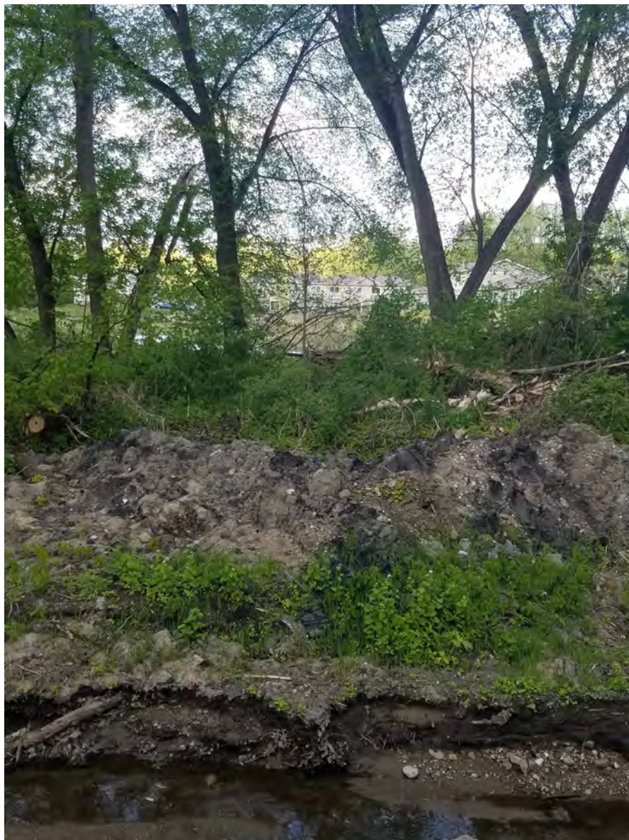
May 6, 2021—Right bank spoils pile and poor vegetation establishment before final grading.
