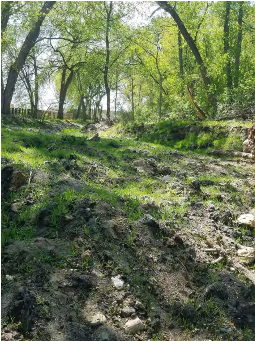
May 6, 2021—Left bank spoil pile and poor vegetation establishment before final grading.
