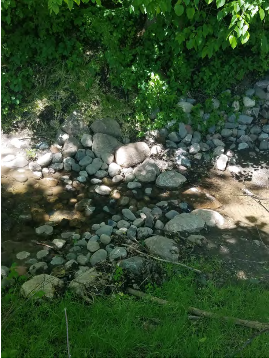
May 28, 2021—Additional riprap placed on right bank; upstream cross vane boulders lowered allowing water to flow more freely.
