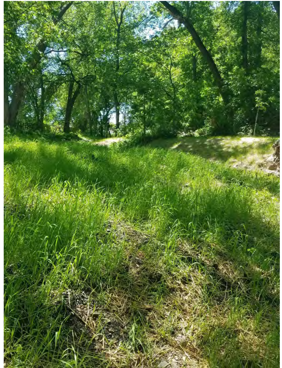
May 28, 2021—Left and right banks re-graded and additional stabilization/erosion control measures installed. Trees planted on upper right bank.
