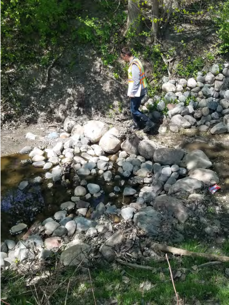
May 6, 2021—Example of right bank erosion at cross vane and incorrect placement of upstream cross vane boulders creating a stagnant pool upstream.
