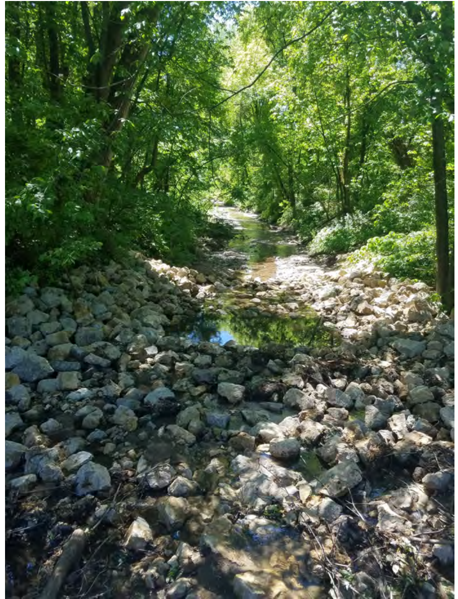
May 28, 2021—Final constructed riprap flume and plunge pool; fallen trees removed from channel.
