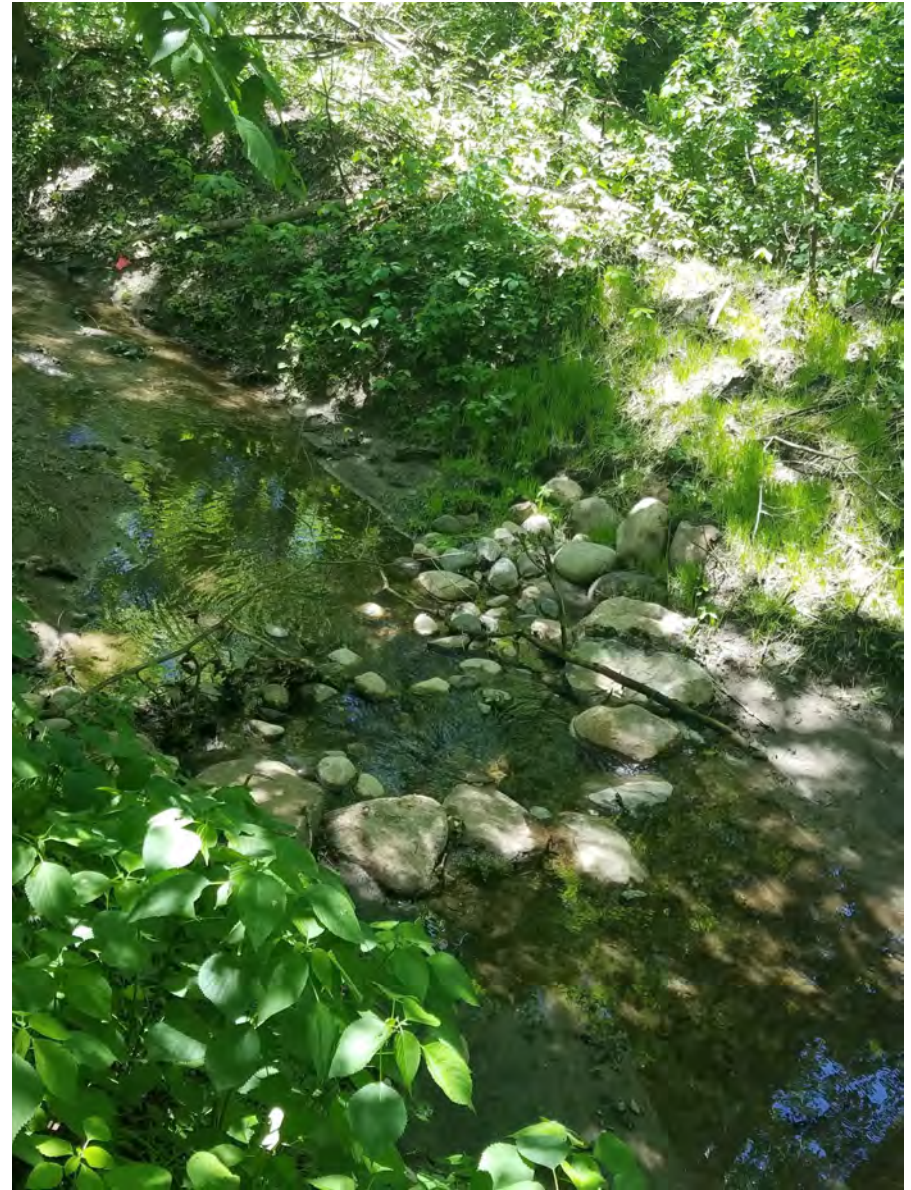
May 28, 2021—Additional riprap placed on both banks, as well as erosion control blanket; upstream cross vane boulders lowered allowing water to flow more freely.
