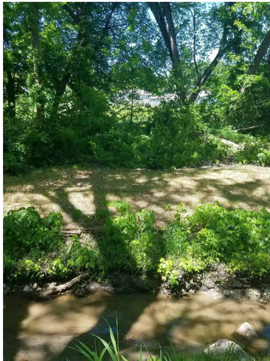
May 28, 2021—Spoils pile removed and erosion control blanket and seeding provided on right bank
