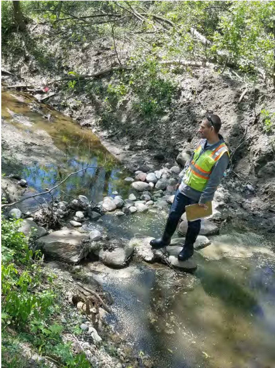
May 6, 2021—Bank erosion at cross vane and incorrect placement of upstream cross vane boulders, creating a stagnant pool upstream.
