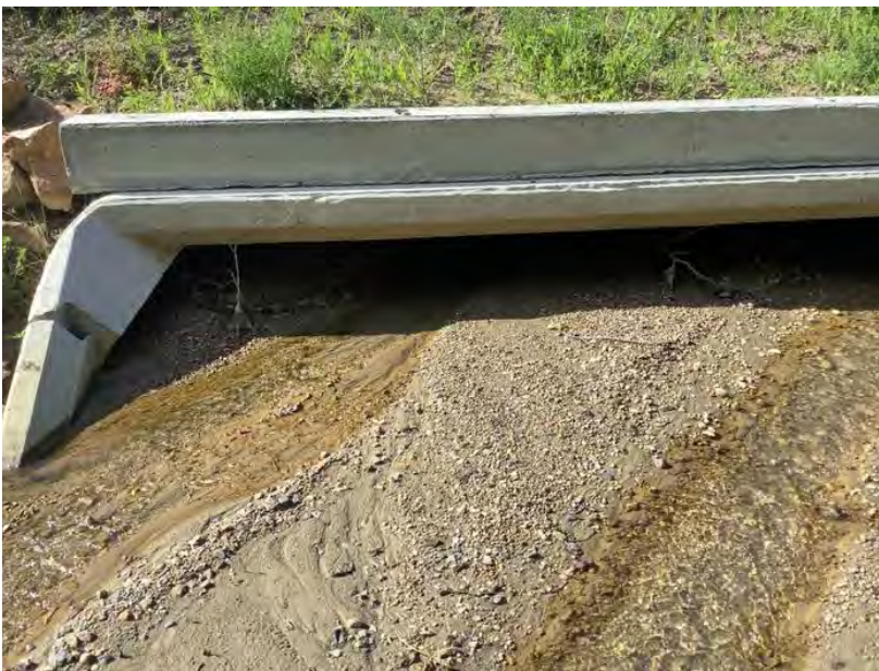
Close up of inlet, some erosion around the apron
