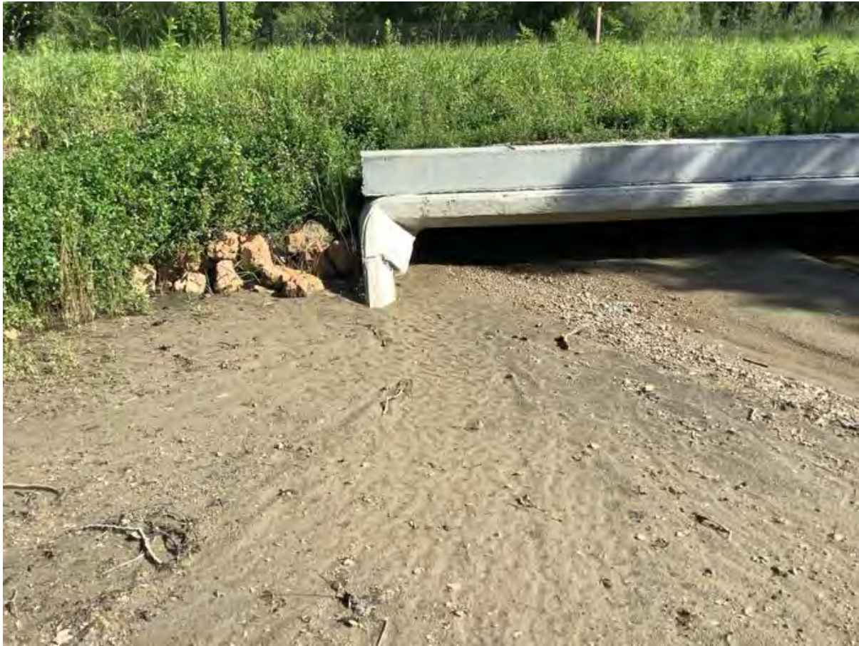
Looking u/s at some erosion along the right apron of the outlet
