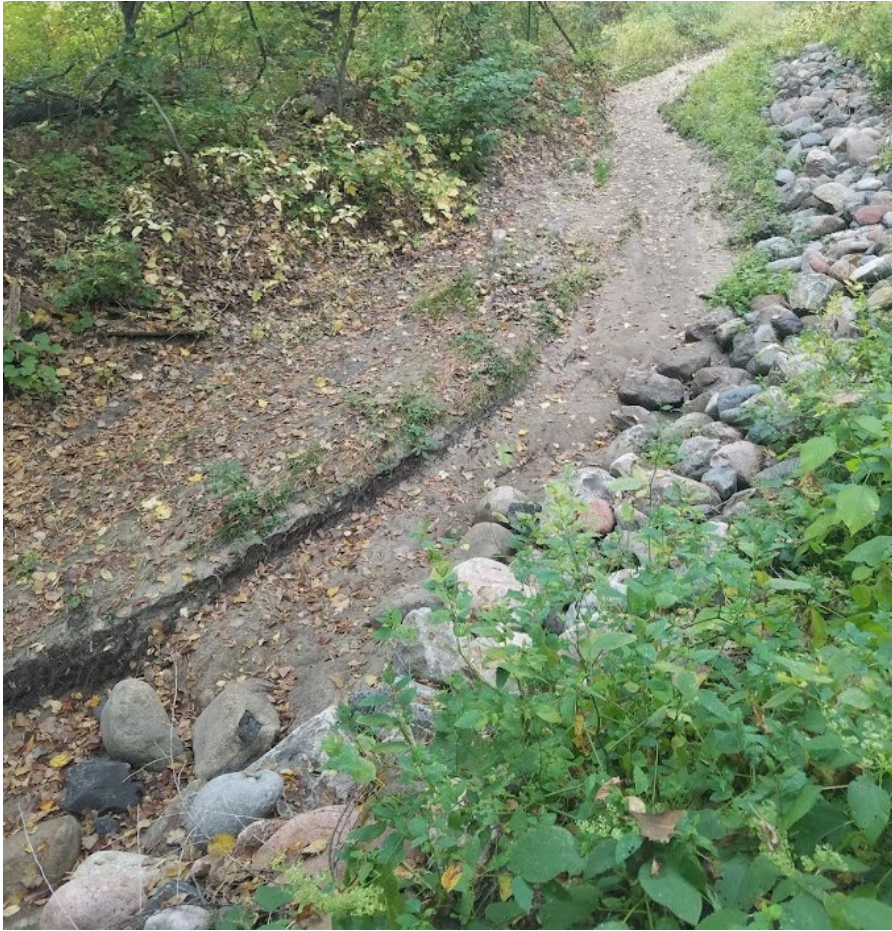
October 2, 2021–Looking upstream at left bank toe protection and established vegetation. Similar amount of erosion is present on the right bank as seen in May 2021.
