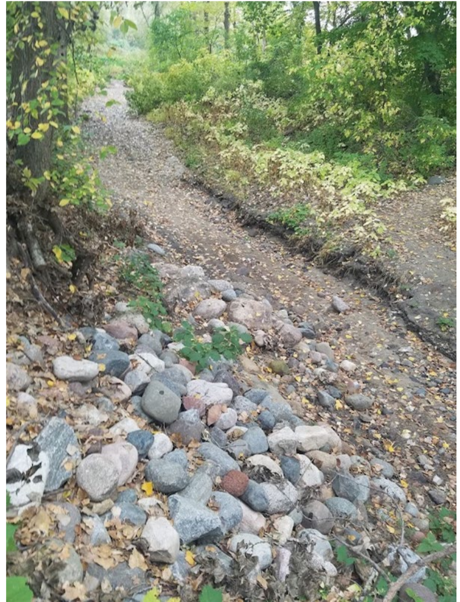
October 2, 2021—Scour within channel at unofficial trail crossing; some slumping of rock material on left bank.
