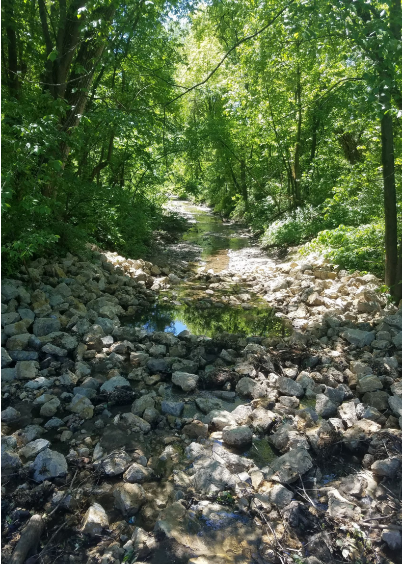
May 28, 2021–Final constructed riprap flume and plunge pool downstream of Crosstown Blvd; fallen trees removed from channel.
