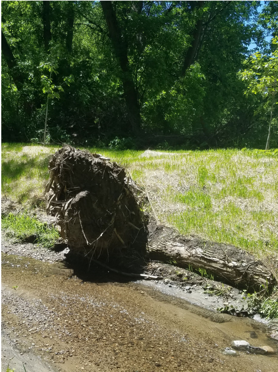
May 28, 2021–Right bank re-graded and additional stabilization/erosion control measures installed. Trees planted on upper right bank.
