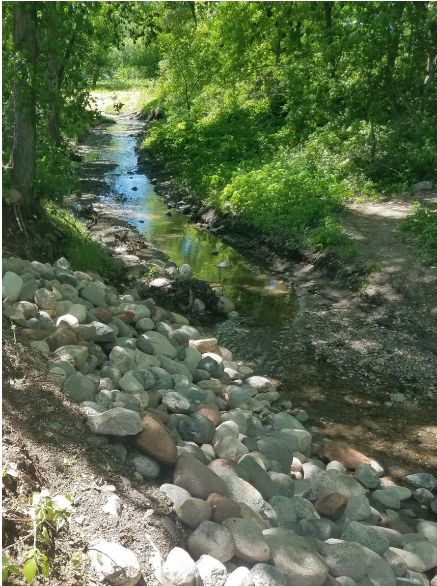
May 28, 2021—Additional riprap placed at area of left bank scour. Existing trail cuts through channel.
