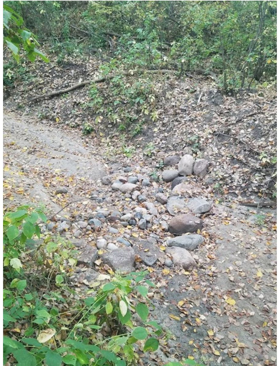
October 2, 2021—Sediment accumulation upstream and downstream of cross vane structure.
