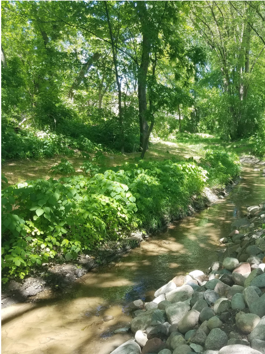
May 28, 2021—Looking upstream at additional grading and erosion control measures placed on right bank.
