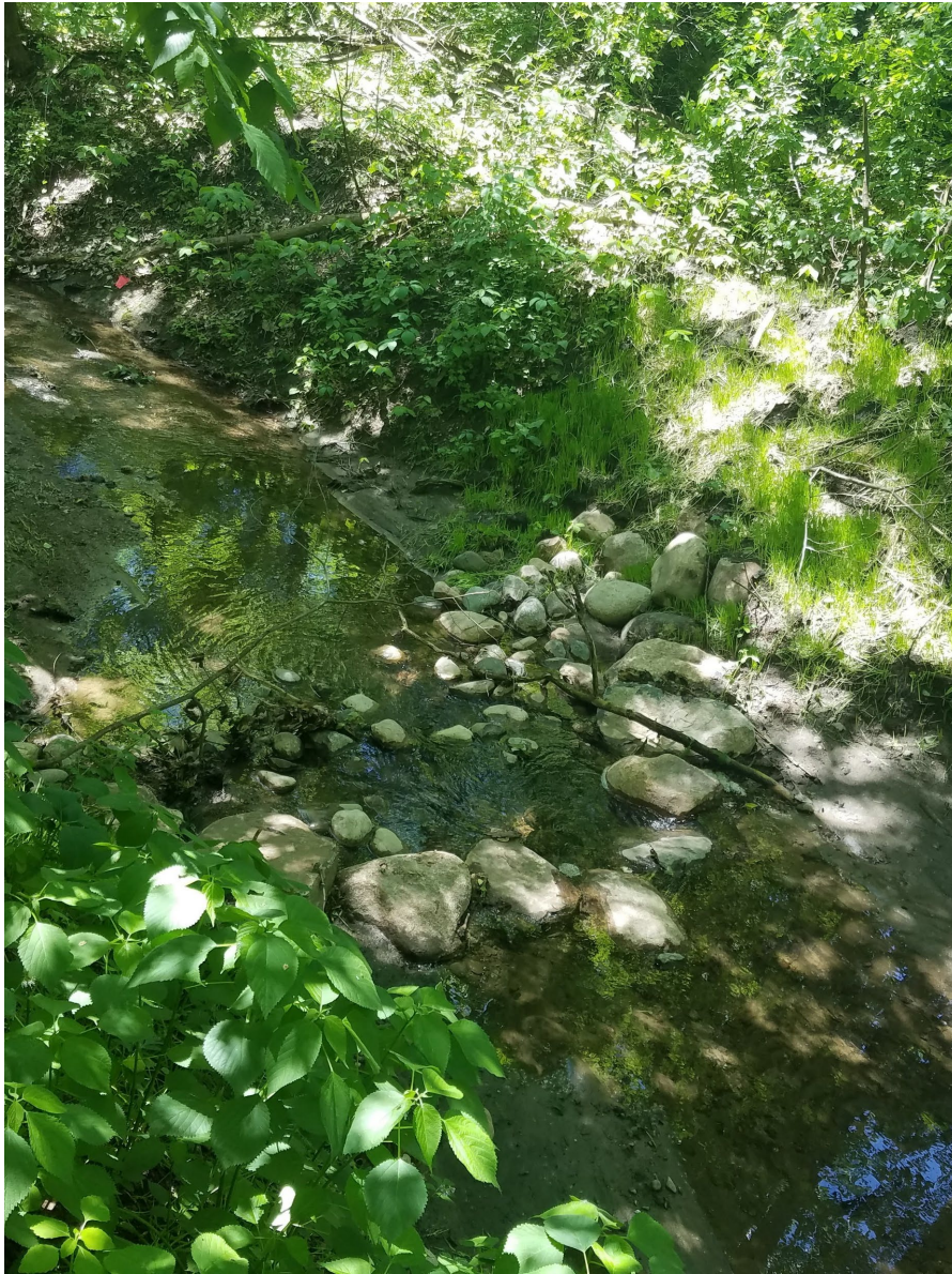
May 28, 2021—Additional riprap placed on both banks, as well as erosion control blanket; upstream cross vane boulders lowered allowing water to flow more freely.
