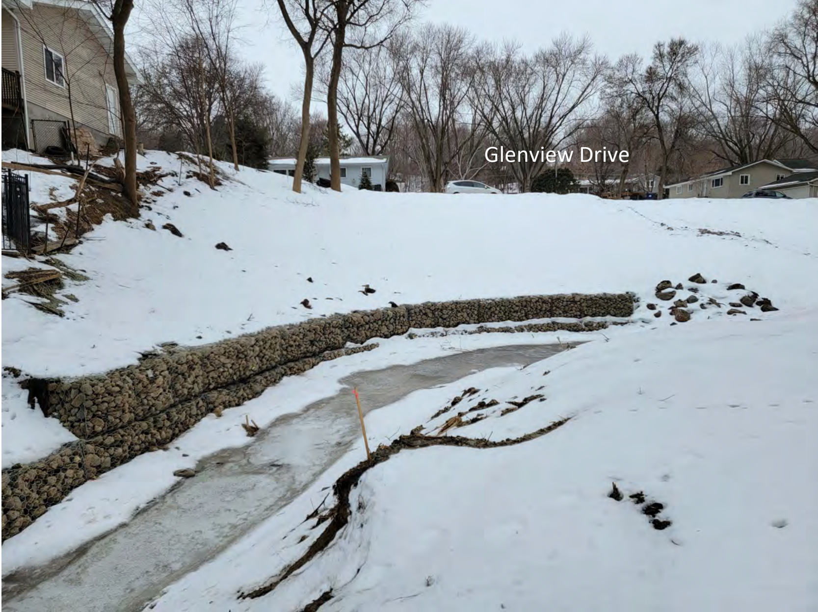
Looking upstream from left bank at gabion toe on right bank and Glenview Drive construction access point
