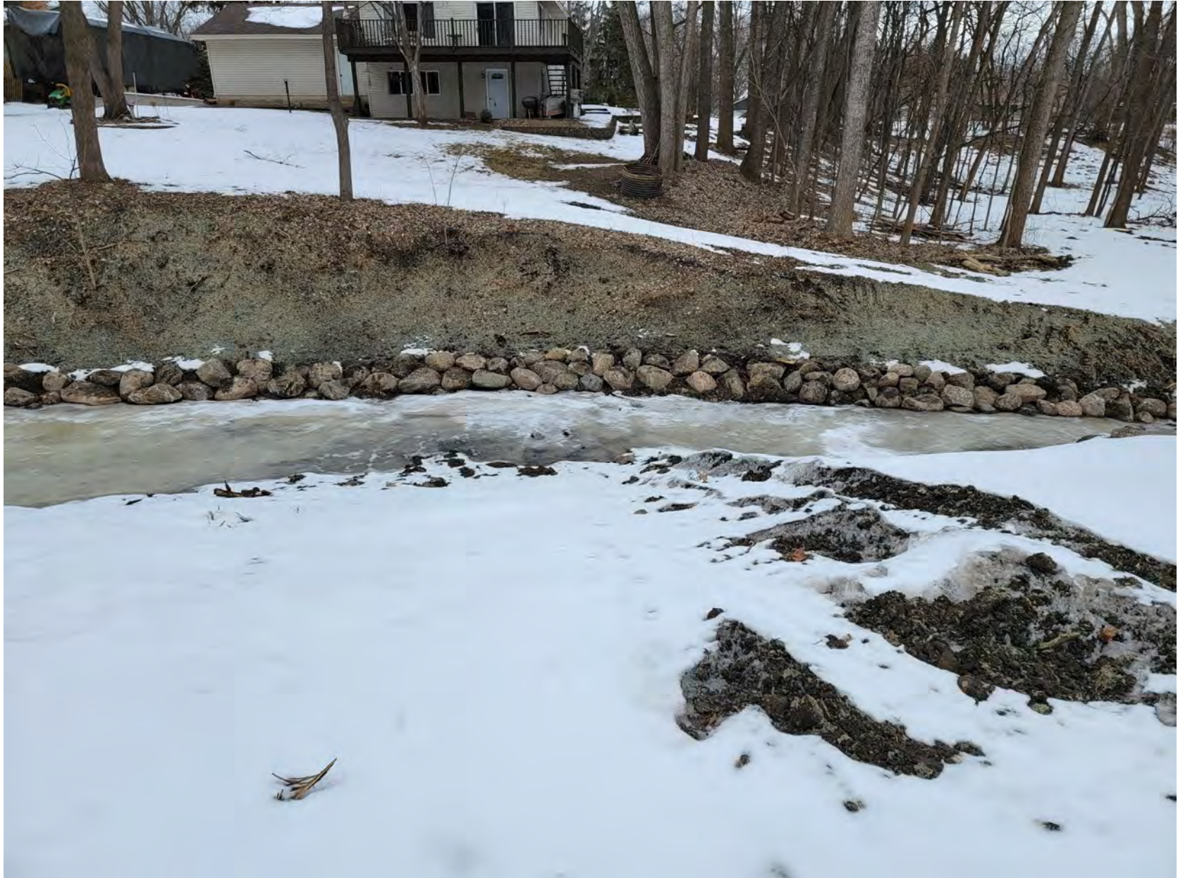
Looking at right bank anchored slope stabilization with rock toe from Glenview Drive construction access point. Appeared to be a sediment delta forming in the channel.
