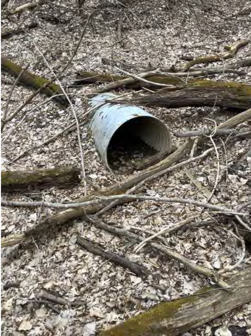
Drainage feature blocked by sticks
