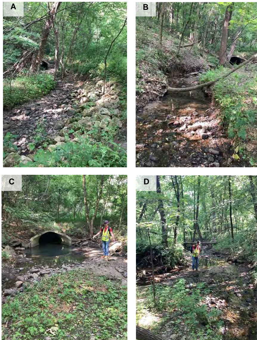
Figure 9: Photos of Gully 06:23-09:32 A) Upstream view of left bank, B) Upstream view of right bank, C) Upstream view of pipe outfall, D) Downstream view of where gully reconnects
