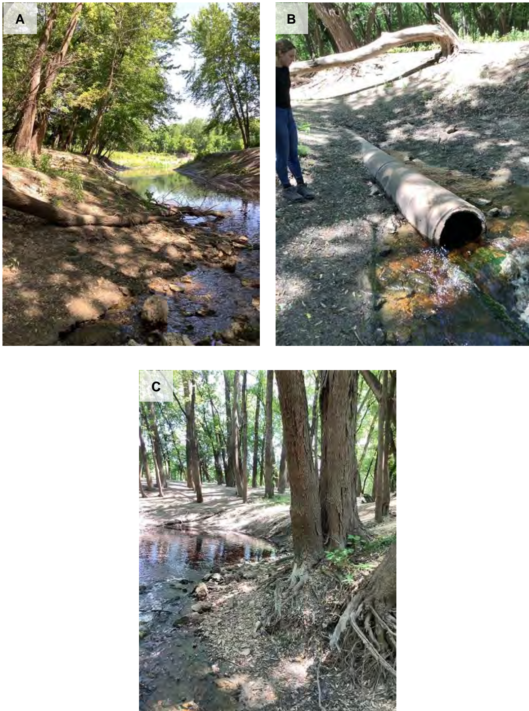
Figure 46: Photos of Gully 06:03-11:34. A) Downstream view of left gully bank, B) Upstream view of pipe with constant, high flow of water exiting the pipe, C) Downstream view of the right gully bank
