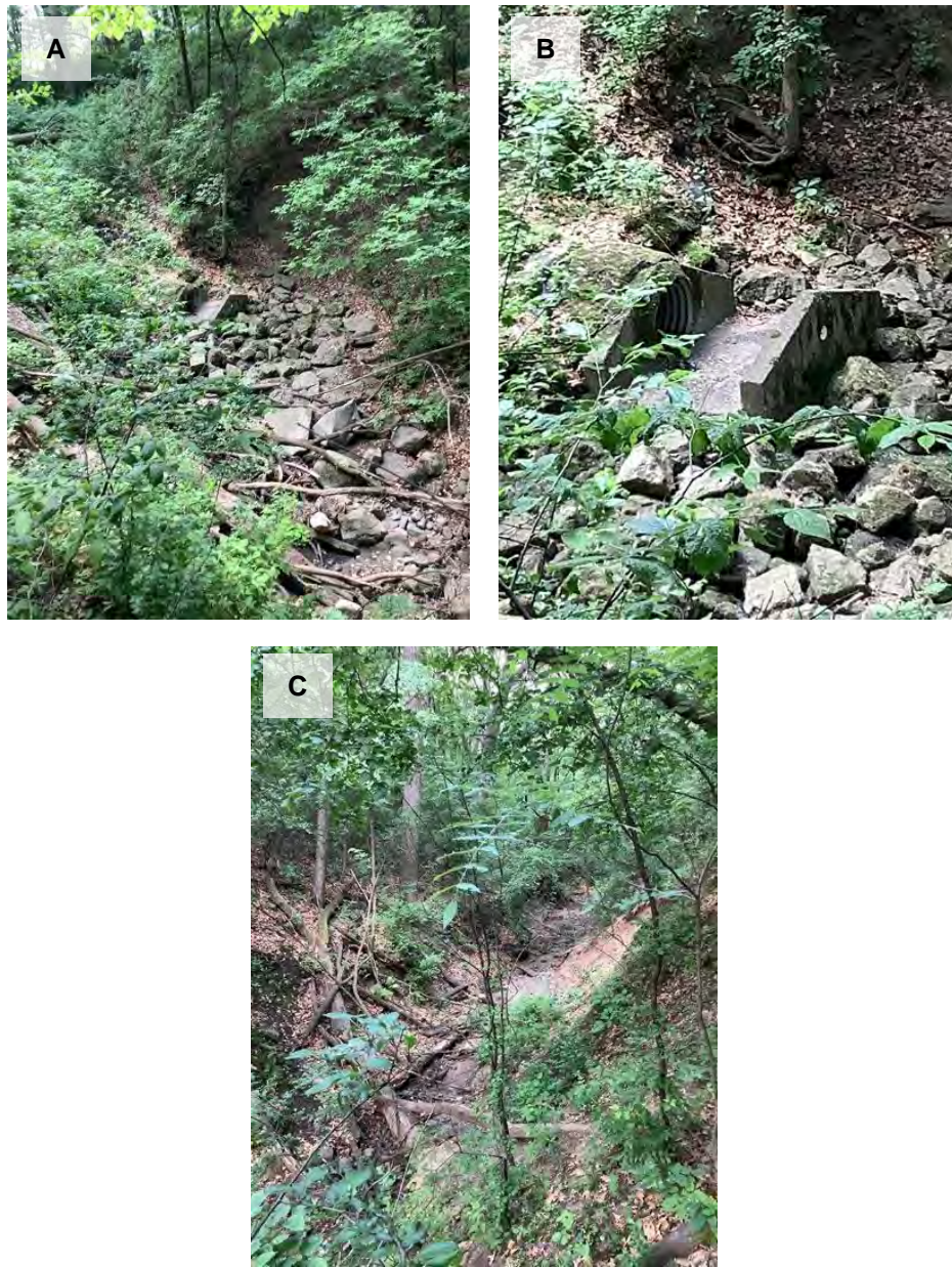
Figure 4: Photos of Gully 06:08-01:06 A) Upstream view of gully, B) Upstream view of pipe, C) Downstream view of gully
