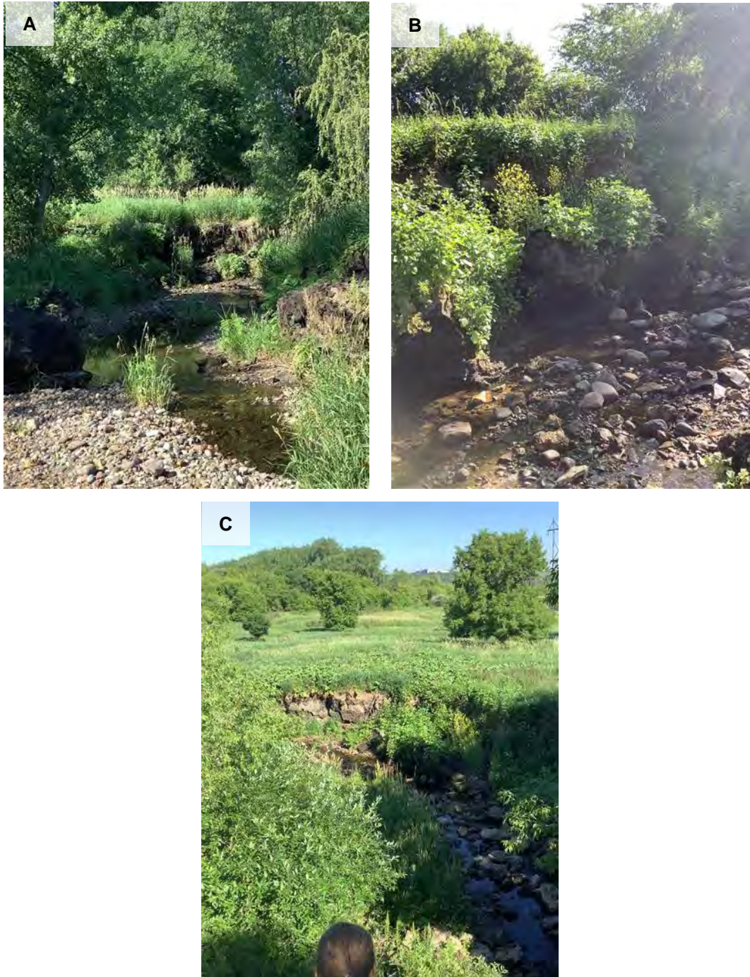
Figure 35: Photos of Gully 06:16-09:07. A) Downstream view of the left bank, B) Upstream view of the right bank showing severe slumping, C) Downstream view of the right bank from a higher perspective
