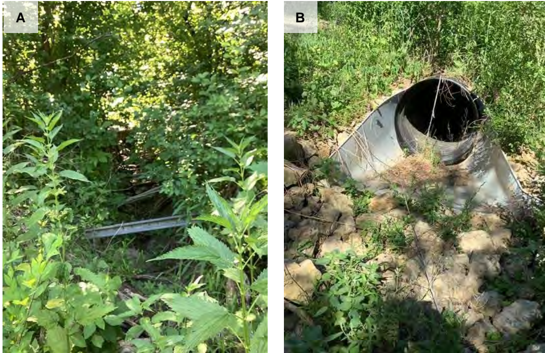
Figure 20. Photos of Gully 06:15-10:06 A) Upstream view of the gully, B) Downstream view of the pipe at the end of the gully
