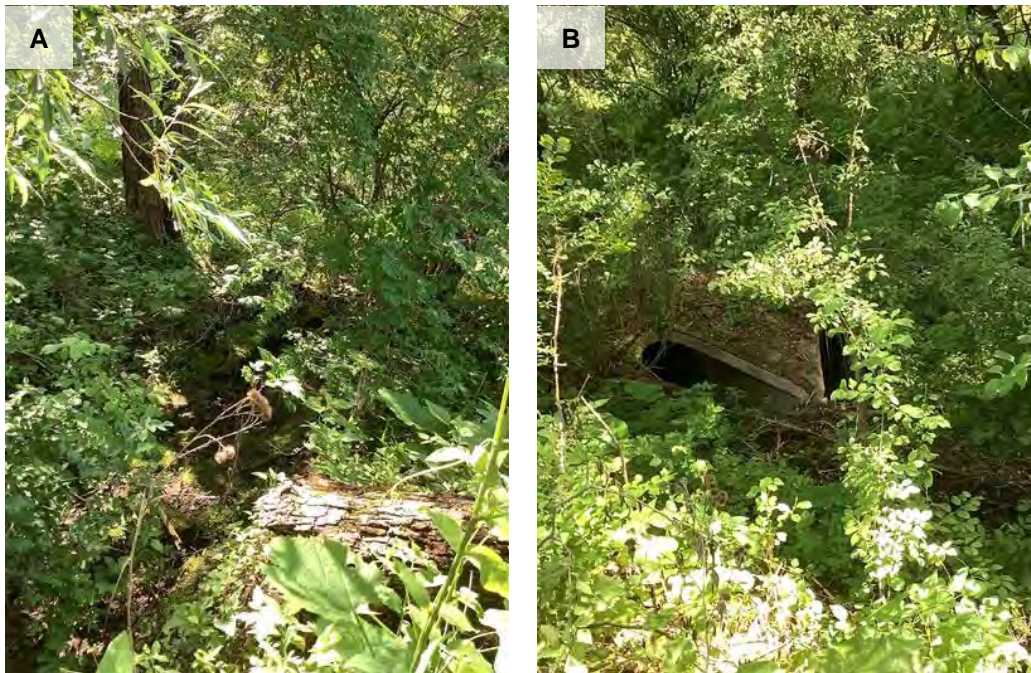
Figure 27. Photos of Gully 06:10-10:04. A) Upstream view of the gully, B) Downstream view of the pipes at the beginning of the gully
