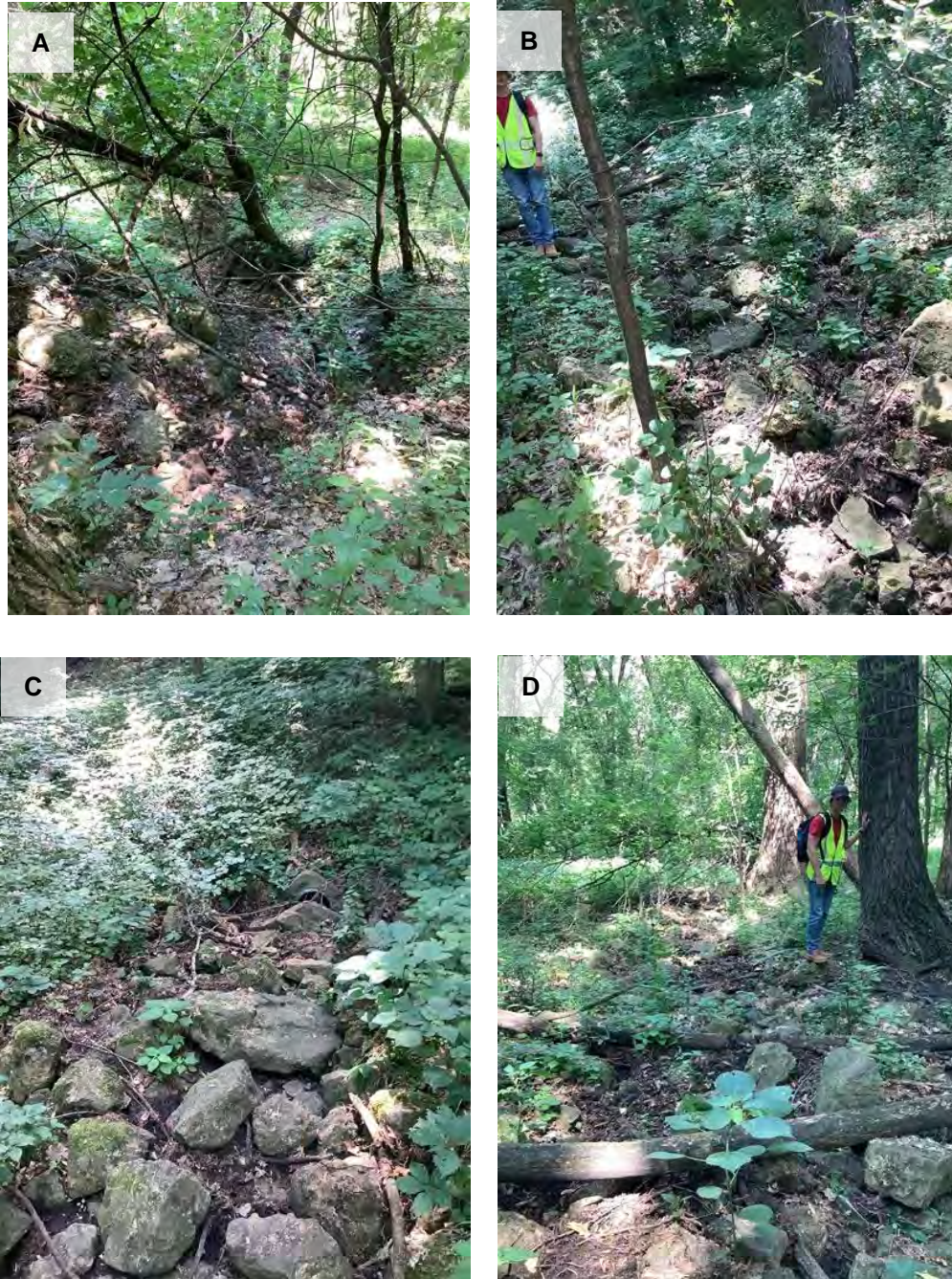
Figure 17: Photos of Gully 06:23-11:37 A) Downstream view of gully, B) Upstream view of gully, C) Upstream view of pipe, D) Downstream view past pipe outfall
