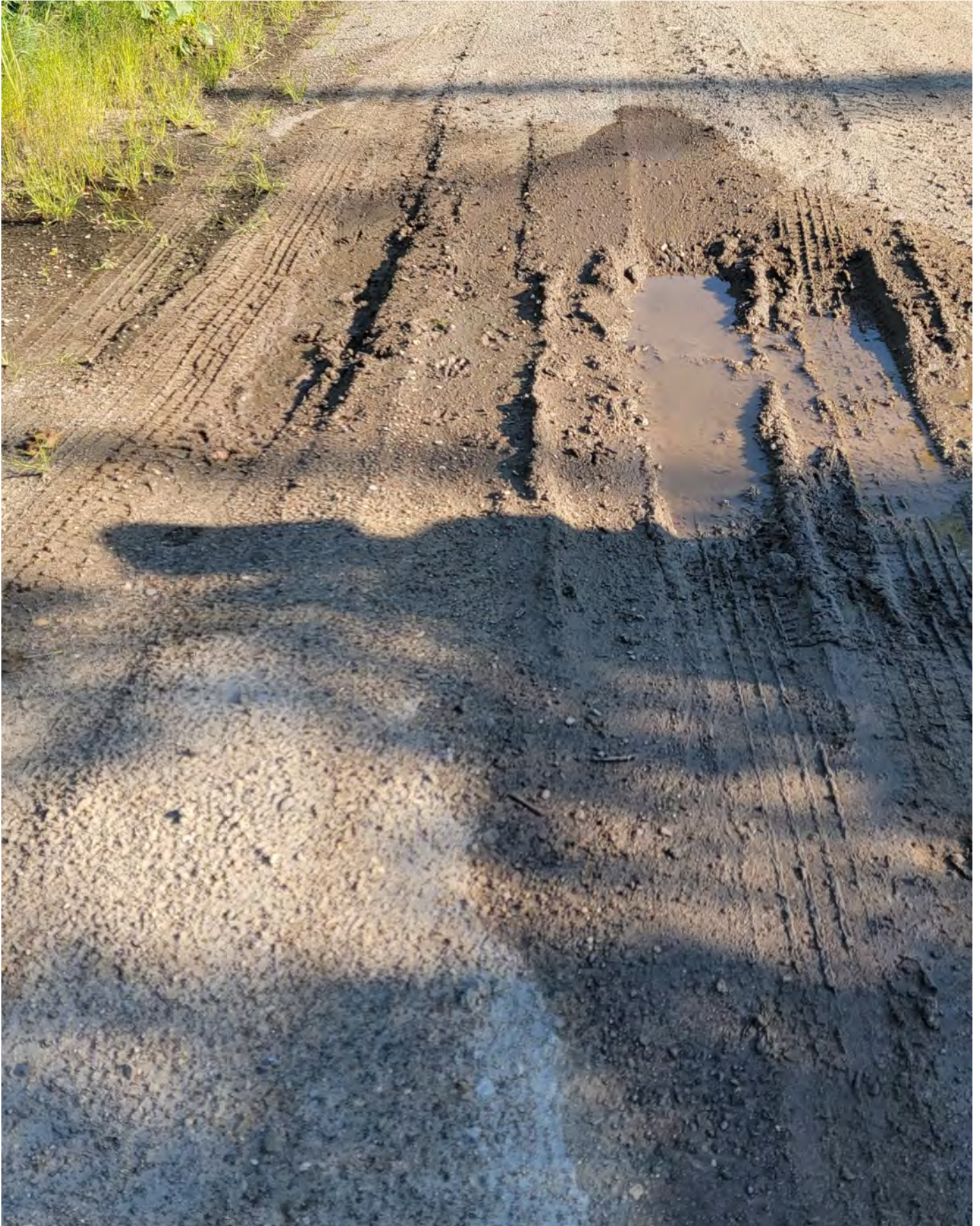
Photo 4B. Close up of rutting and pavement condition, looking north
