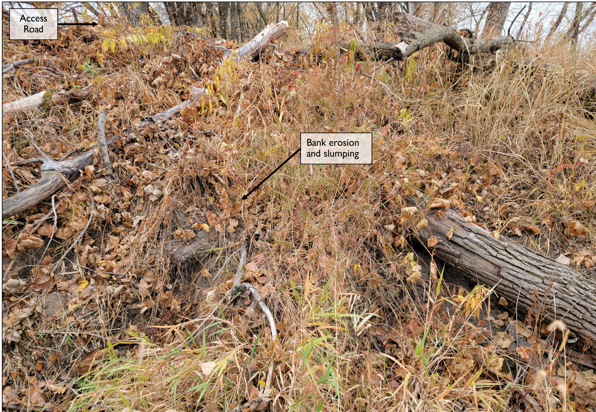
2. Looking north at upstream embankment from above the presumed culvert alignment at debris and inslope erosion.
