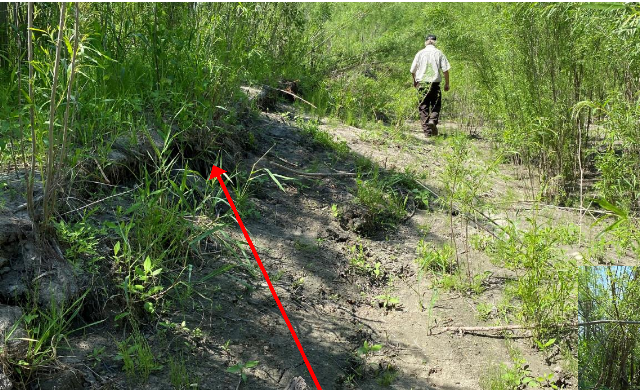
Evidence of Sloughing of Natural Levee
