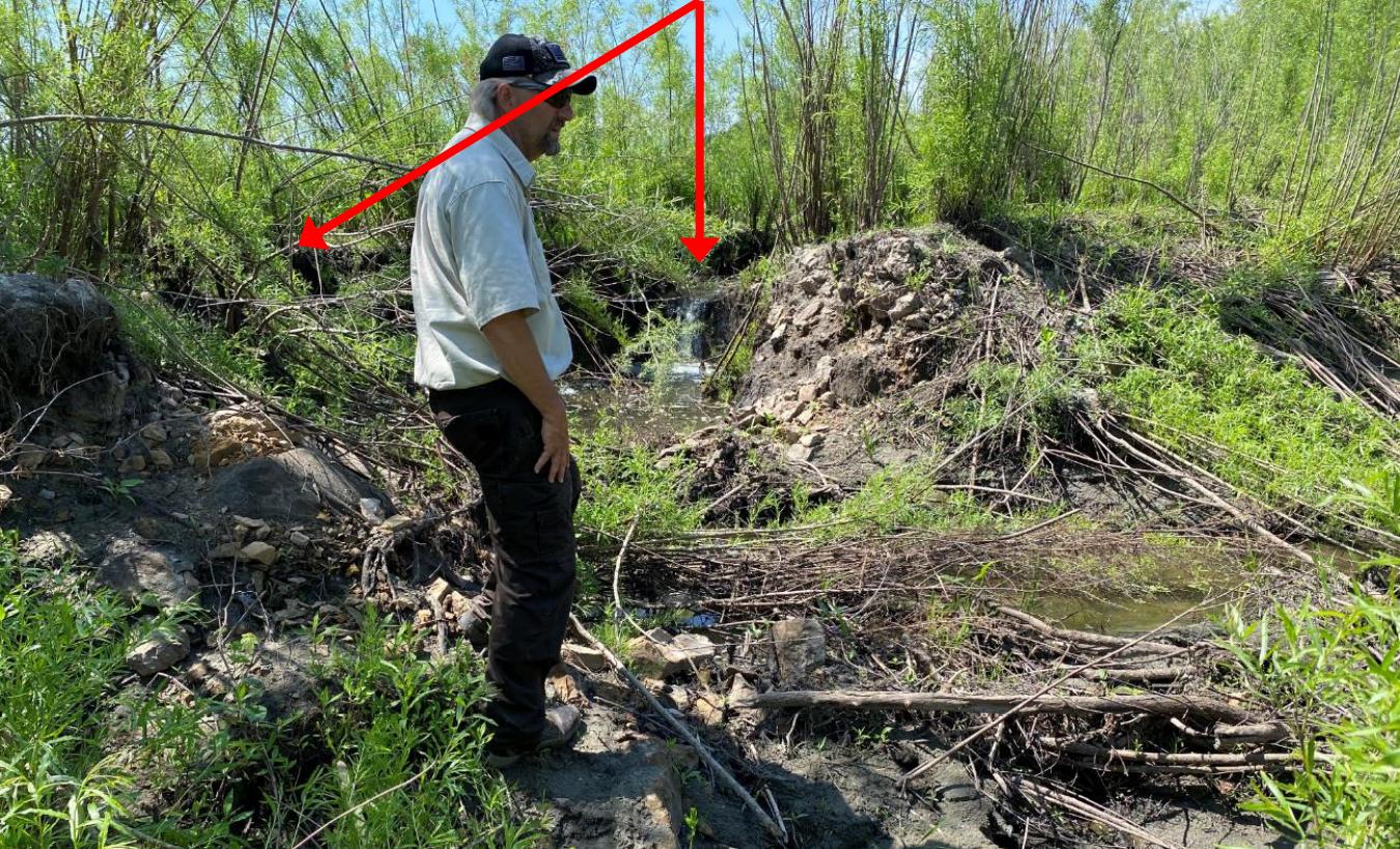
Breach of Natural Levee
