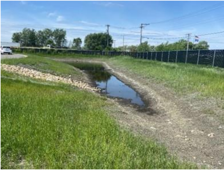
Photo 1 Violation - Lack of vegetation establishment throughout pond exterior
