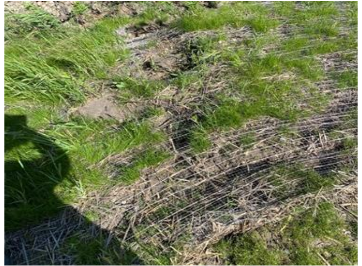
Photo 4 Violation - Undermining of erosion control blanket and subsequent hillslope erosion
