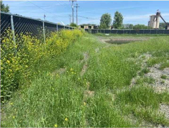
Photo 3 Violation - Erosion and lack of vegetation establishment leading from southwest corner of site to pond
