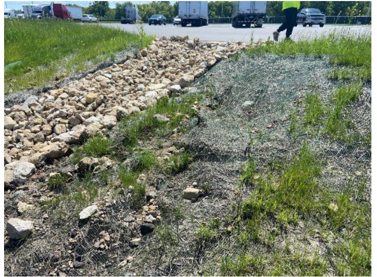
Photo 2 Violation - Erosion and gulying adjacent to rip rap channel leading to pond
