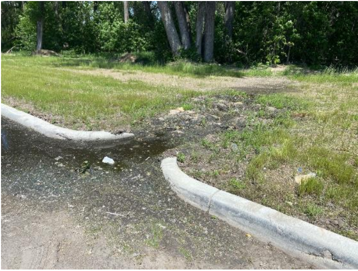
Photo 1 Violation - Rip rap at northeast curb cut clogged with sediment and debris, preventing drainage
