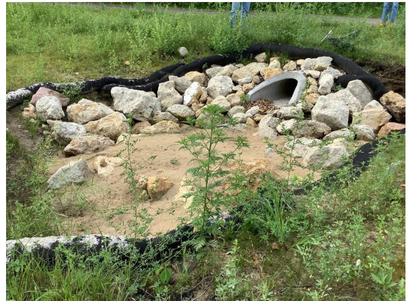
Figure 4: Sediment in Stormwater Outlet at Xcel Driveway
