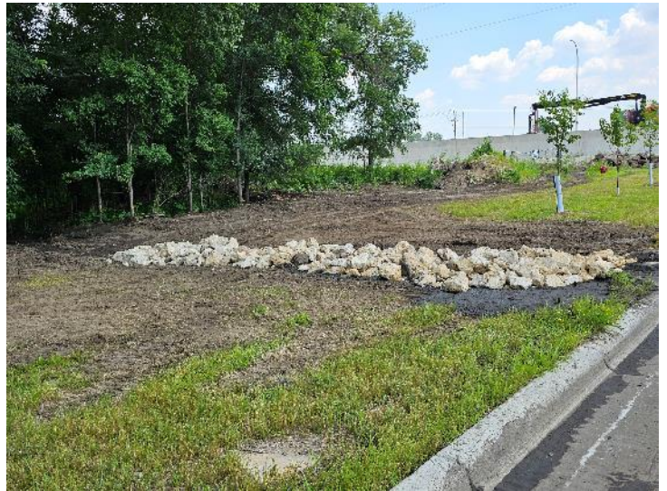
Photo 4 Correction - Rip rap cleaned, additional rip rap installed, and regrading at northeast curb cut
