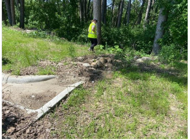
Photo 2 Violation - Rip rap at northwest curb cut clogged with sediment and debris
