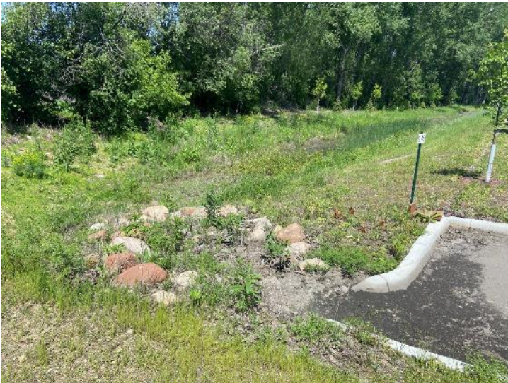
Photo 3 Violation - Rip rap at southwest curb cut clogged with sediment and debris
