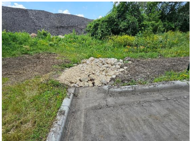
Photo 6 Correction - Rip rap cleaned, additional rip rap installed, and regrading at southwest curb cut
