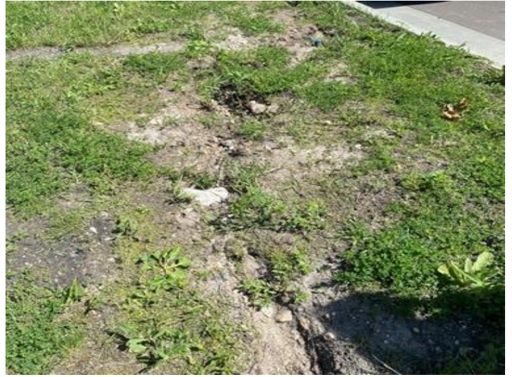
Photo 2 Violation - Gully erosion observed downslope from catch basin
