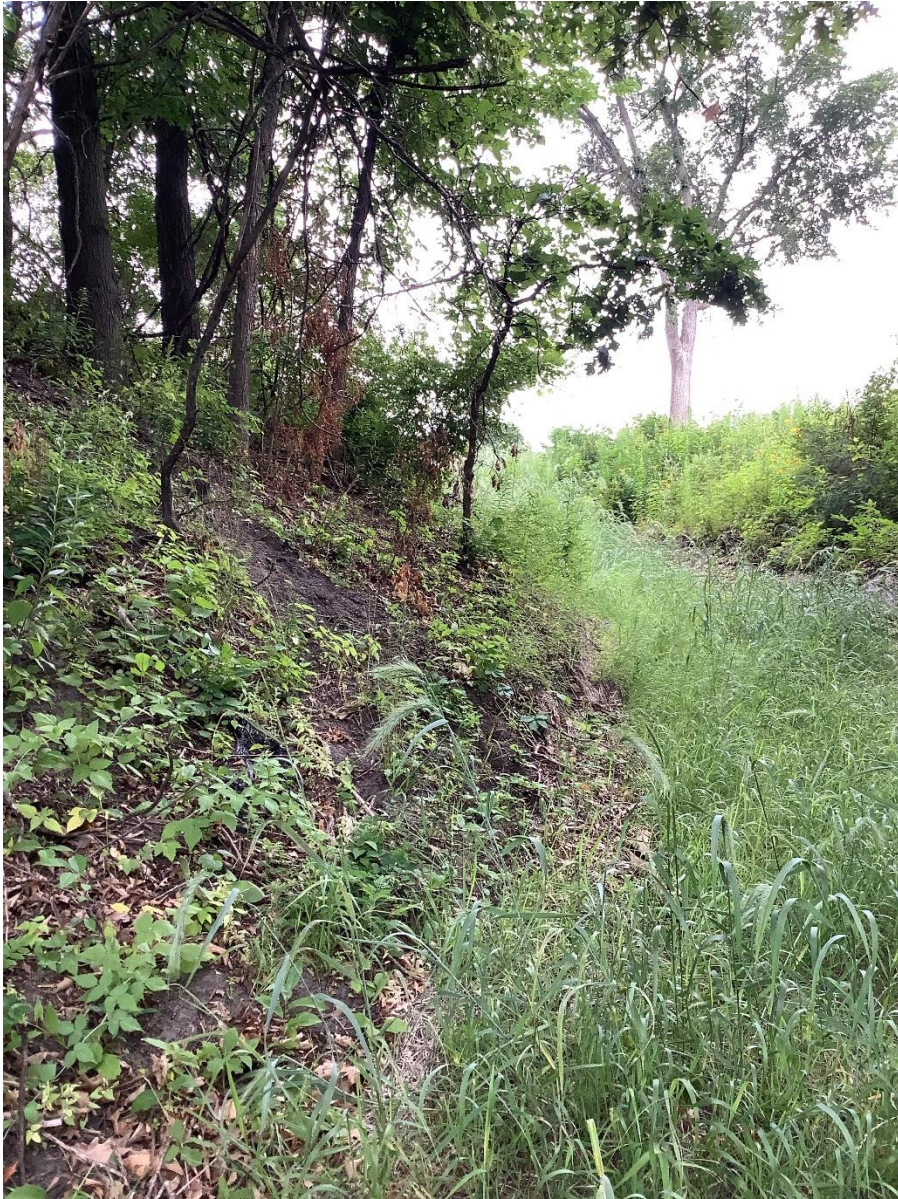
Figure 3: Eroding Slope at Eagle Creek Bridge
