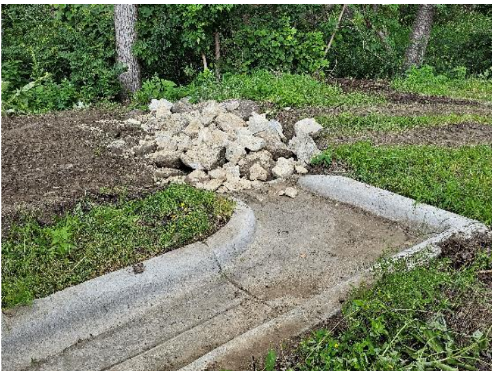
Photo 5 Correction - Rip rap cleaned, additional rip rap installed, and regrading at northwest curb cut
