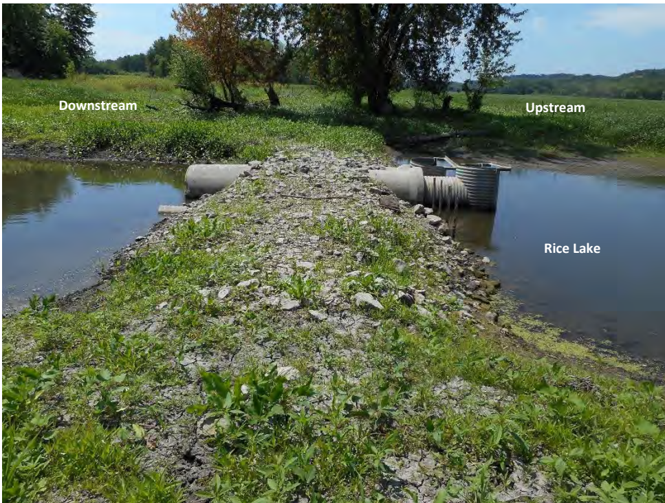
Field Road Over Outlet Pipes at Rice Lake Outlet Looking South (photo taken 7/17/17)
