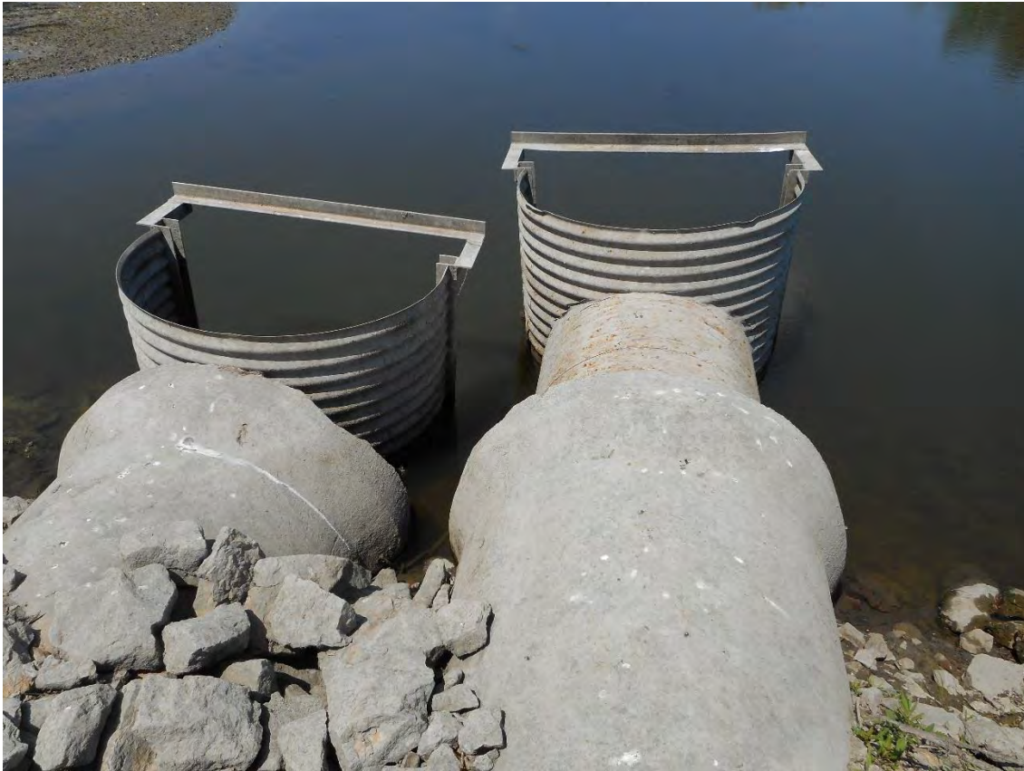
36-inch Concrete Outlet Pipes with Stoplog Weirs at East End of Rice Lake Looking Northwest (photo taken 7/17/17)
