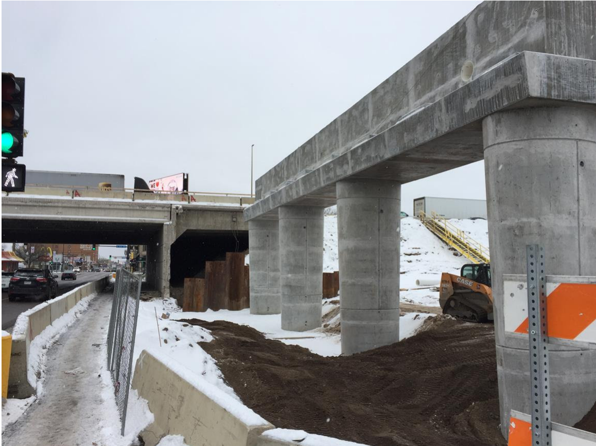
Looking east, bridge piers rise at the future I-35W & Lake Street Station
