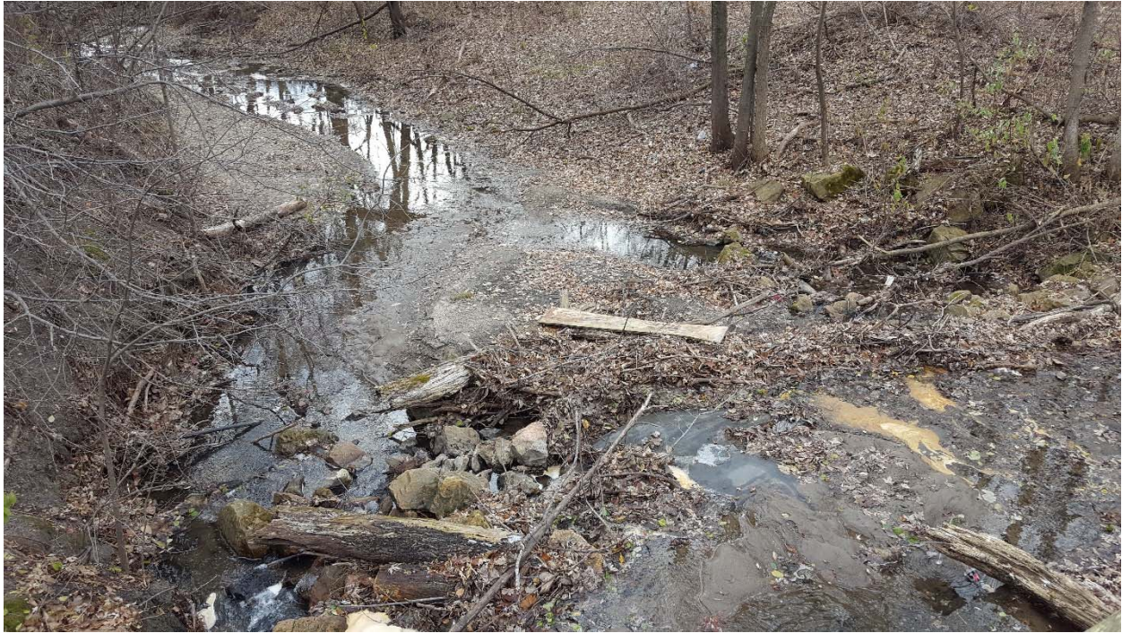
Photo 11: Site S1 – scour hole and erosion downstream of Crosstown Boulevard
