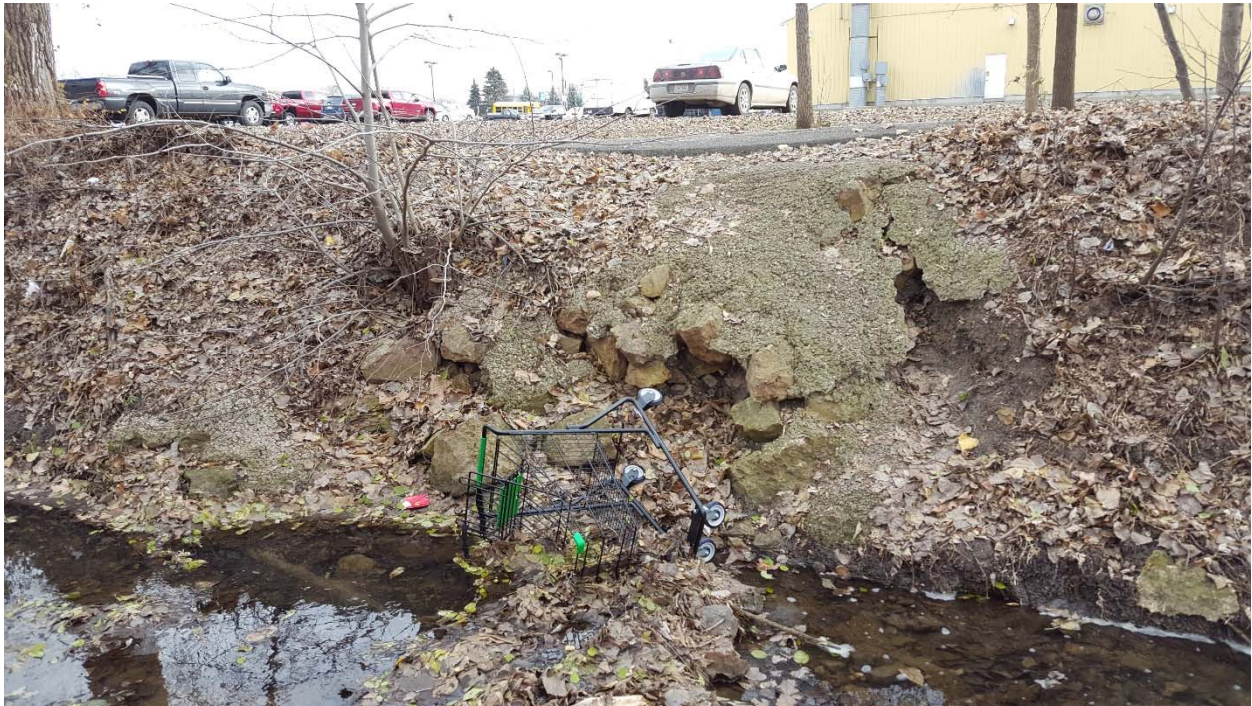
Photo 14: Site S4 – eroding bank and debris in the channel
