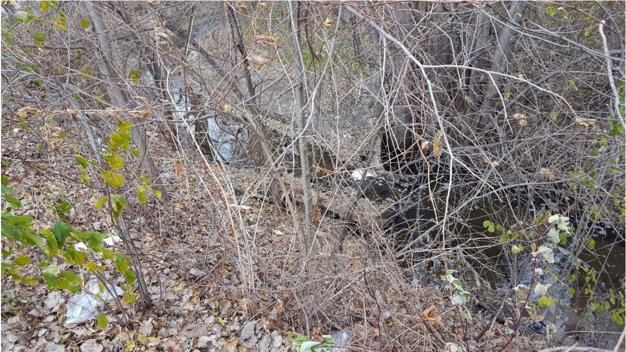
Photo 4: Site M7 – debris in channel causing blockage
