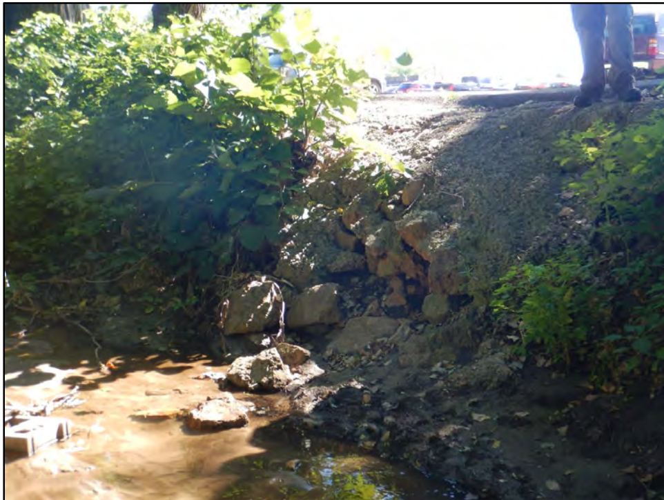
Photograph B-10: View east of bank erosion.
