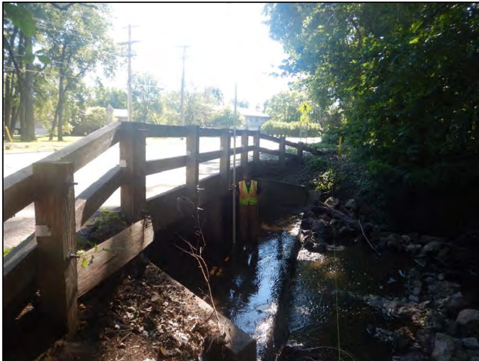
Photograph B-3: View southeast of bridge crossing and scour hole.
