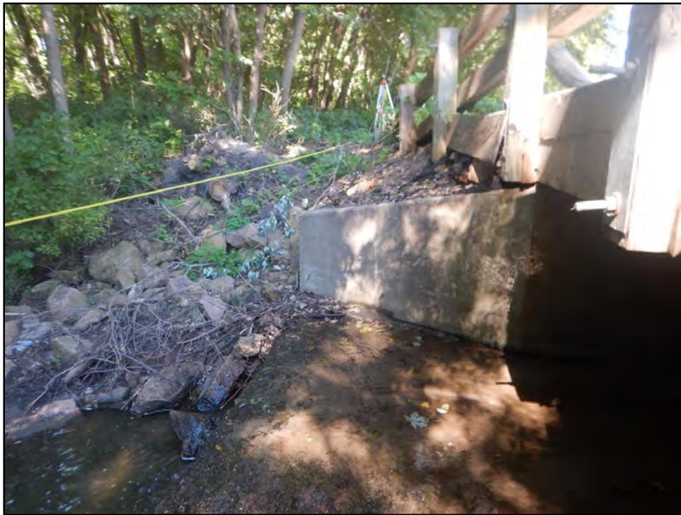
Photograph B-5: View northwest of scour hole.
