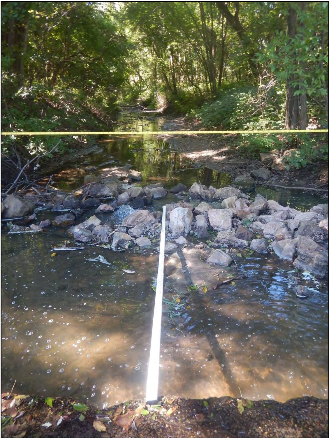
Photograph B-4: View southwest of scour hole.
