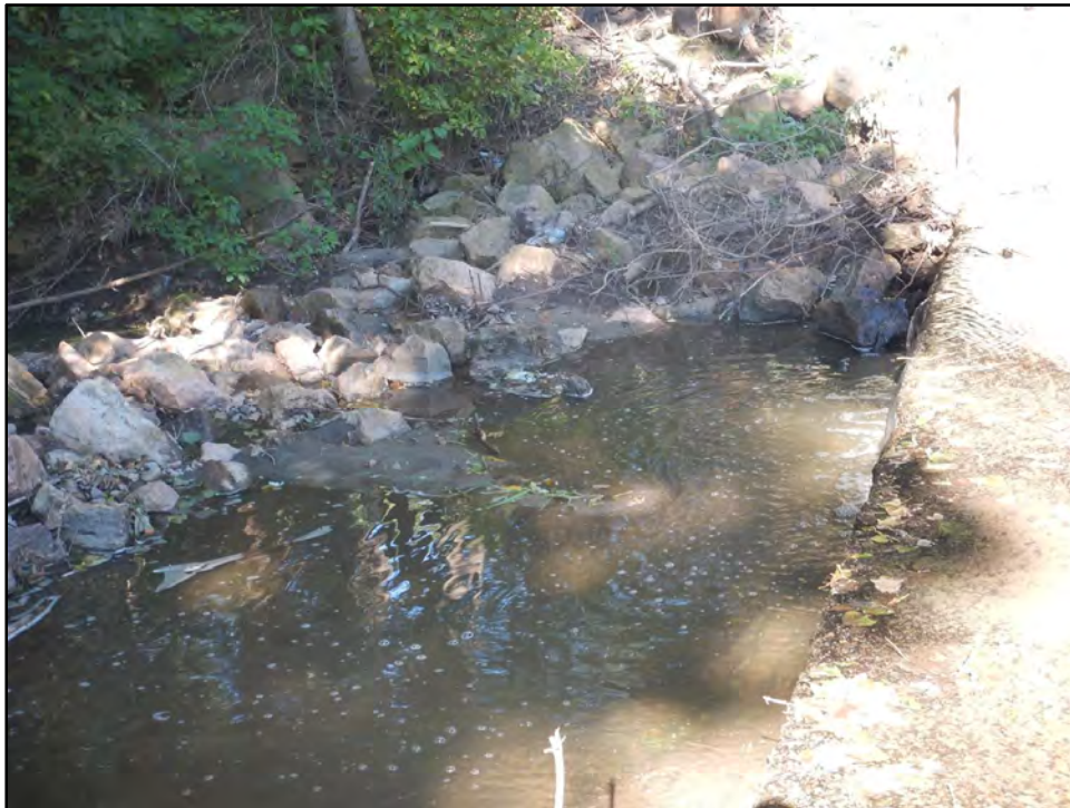
Photograph B-1: View northwest of scour hole.
